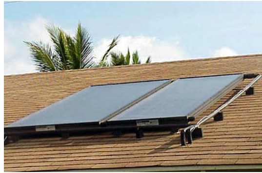
Flush mounted solar hot water panels
