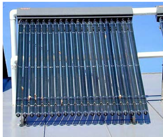
Evacuated tube collectors
